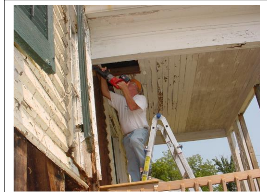
Ray Carney works to stabilize a deteriorated beam in order to lock the double doors.
